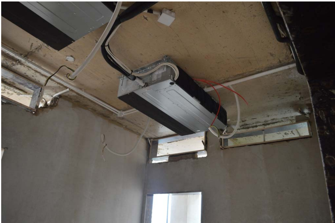
Figure 24: Mechanical installations on 9th floor
