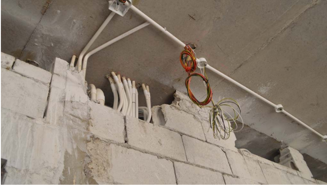
Figure 21: Electrical installations in 11th floor
