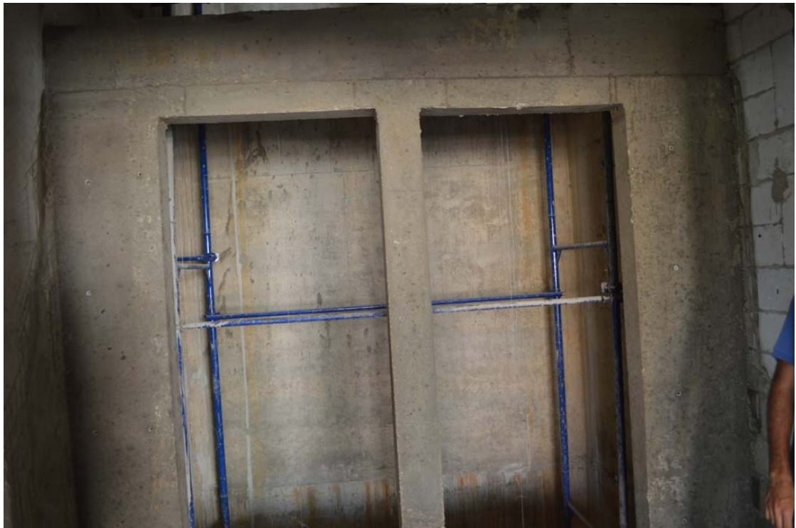
Figure 22: Elevators ready for next step
