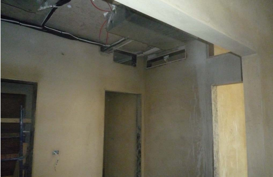
Figure 45: Fan coil units installed @ 3rd floor
