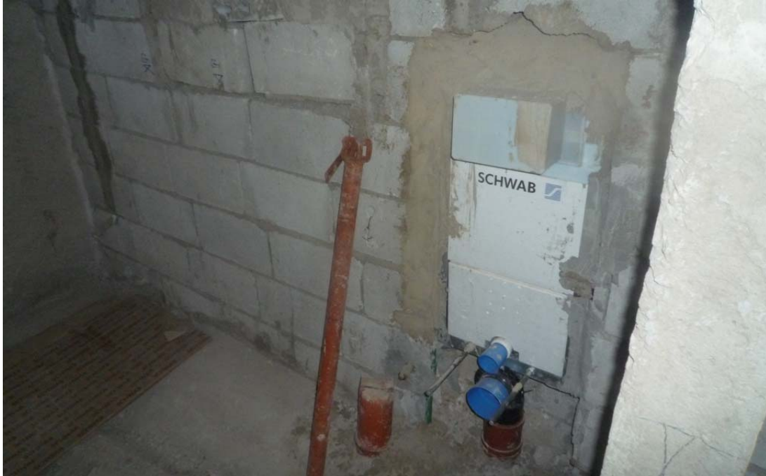
Figure 31: Plumbing installations @ 9th floor
