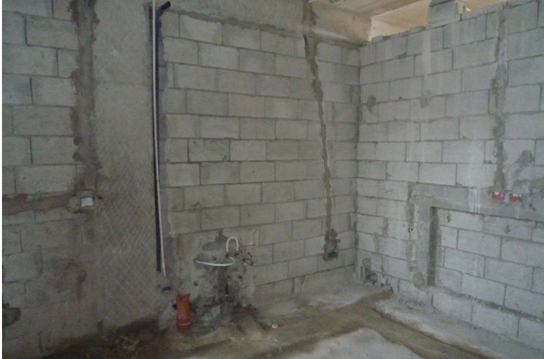
Figure 27: Kitchen plumbing installations @ 10th floor
