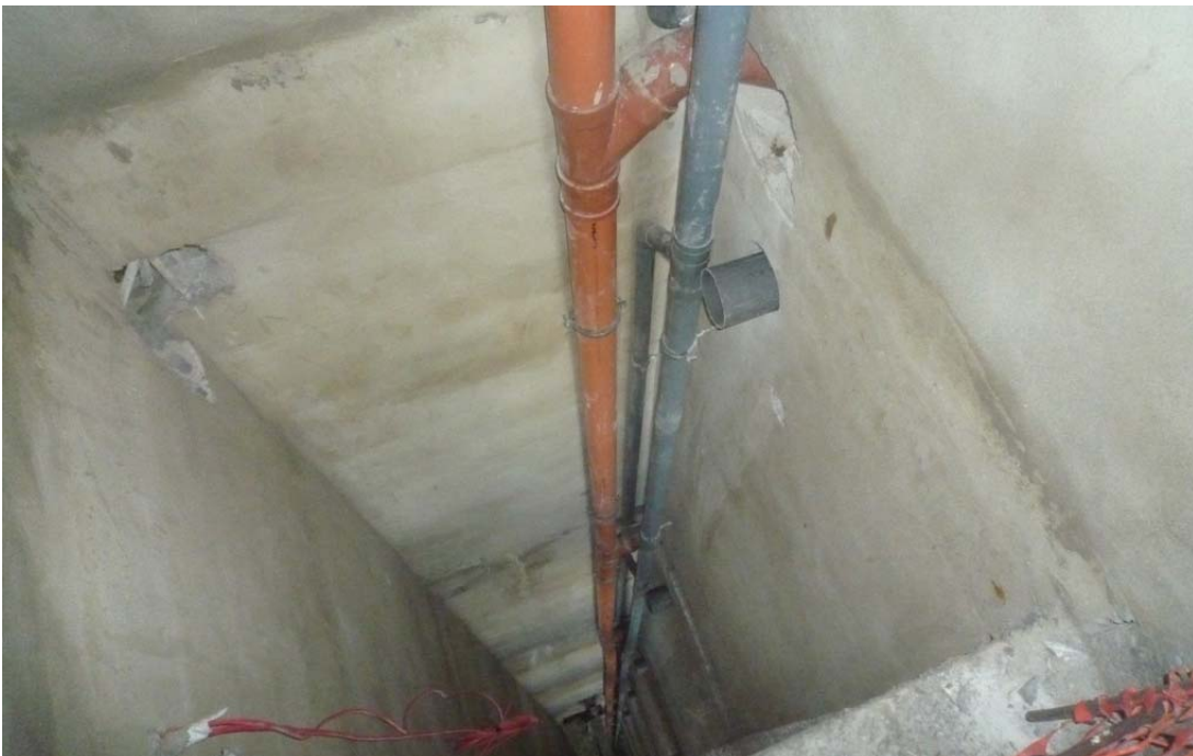
Figure 26: Mechanical installations in shaft / view from the 10th
