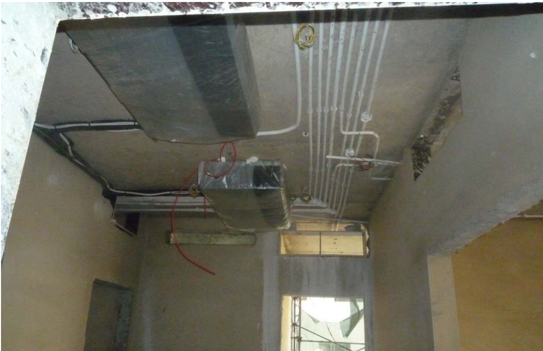
Figure 44: Fan coil units installed @ 3rd floor
