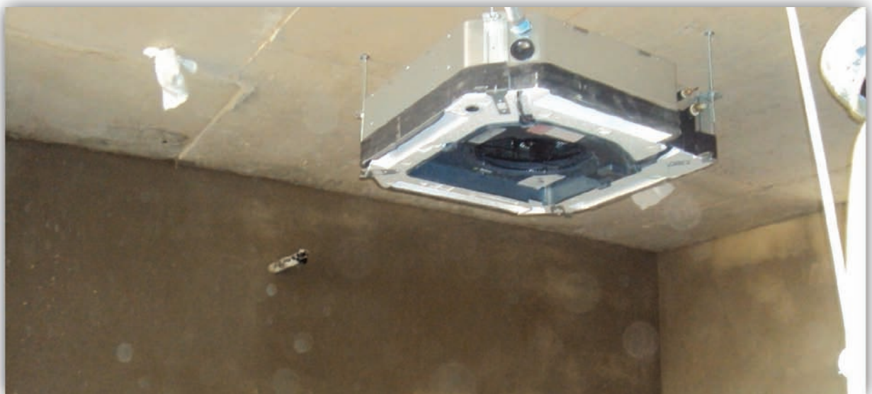
Figure 36: Mechanical installations in 2nd floor (kitchen) - June 2012
