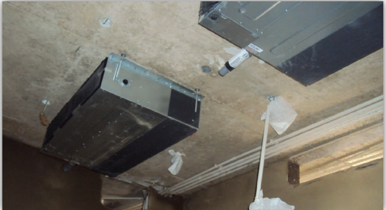
Figure 35: AC indoor units installed in 2nd floor - June 2012
