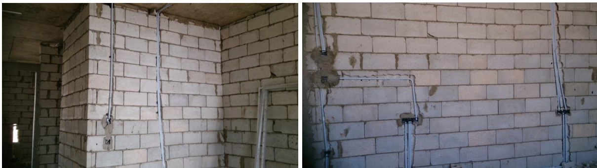
- Electrical pipes in 13 th floor .
