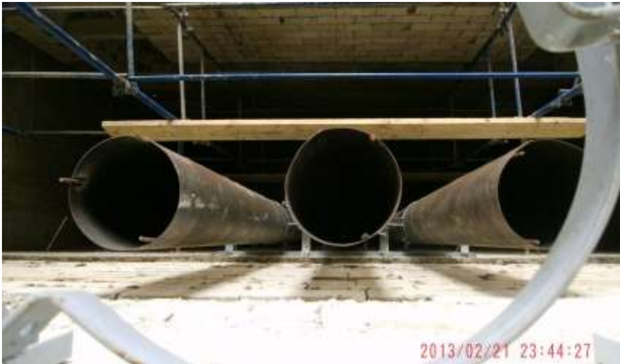
- Generators exhausts up to 14 th floor.
