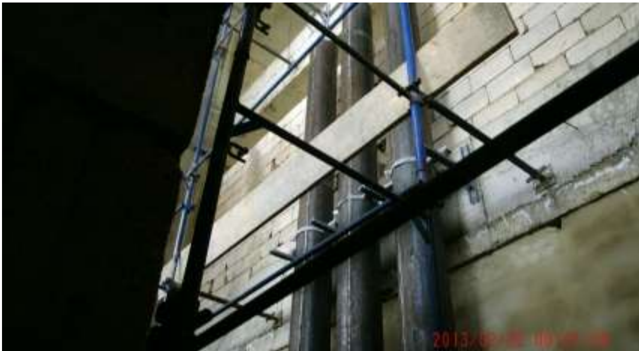
- Generators exhausts up to 14 th floor.
