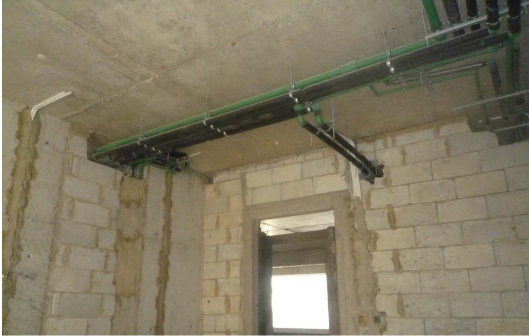
Figure 32: Plumbing installations @ 7th floor
