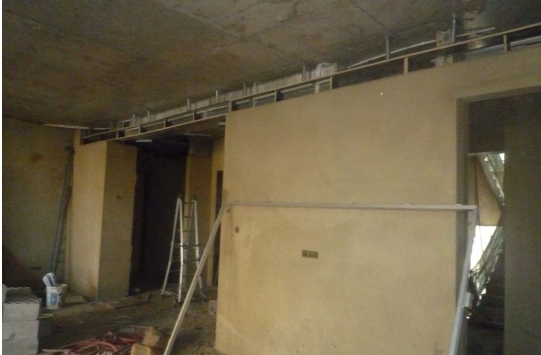
Figure 28: Air outlets @ 3rd floor
