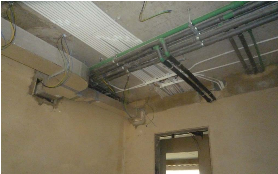
Figure 15: Electrical and mechanical installations @ 1st floor
