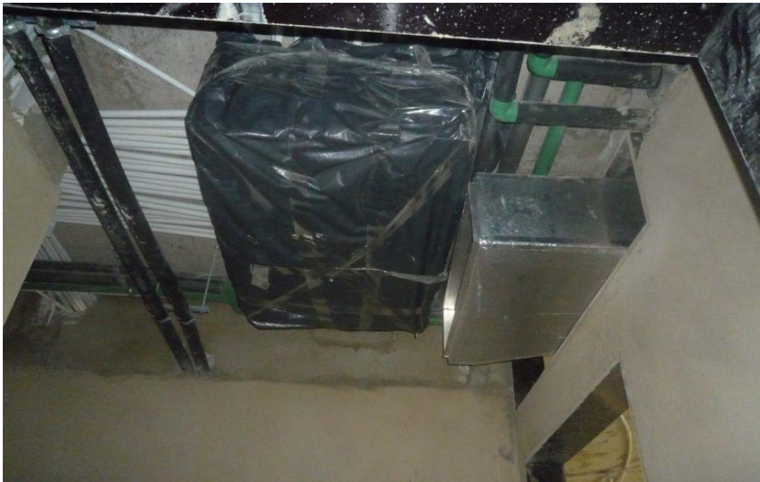
Figure 29: Fan coil units installed @ 2nd floor
