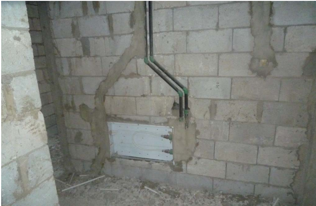
Figure 33: Floor heating manifold installed @ 6th floor
