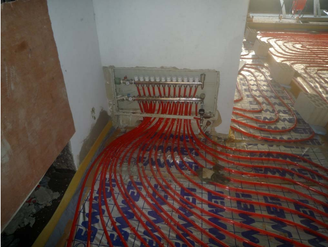
Figure 13: Underfloor heating manifold installed @ 1st floor
