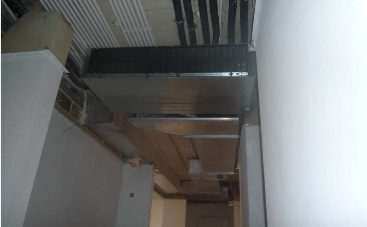
Figure 11: Fan coil units installed in 1st floor
